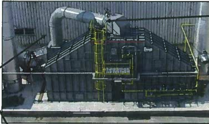
REFRACTORY LINED DAMPER
